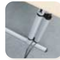
Vertical cable riser
